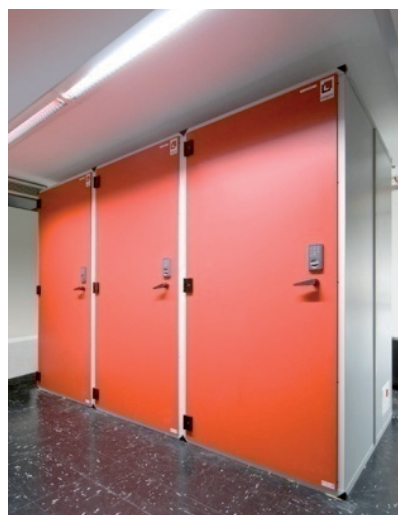
Figure 2. City of Marburg data center.
