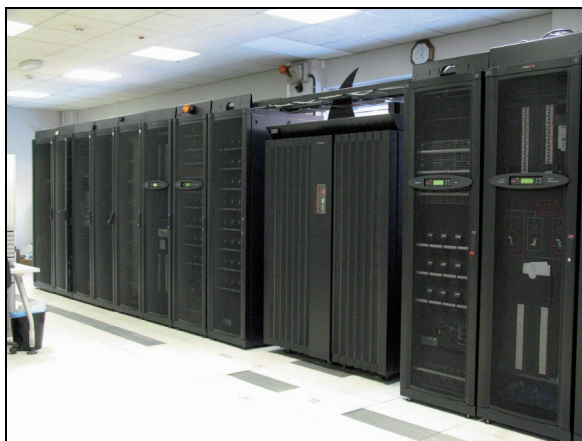
Figure 1. Data center zone 2.
